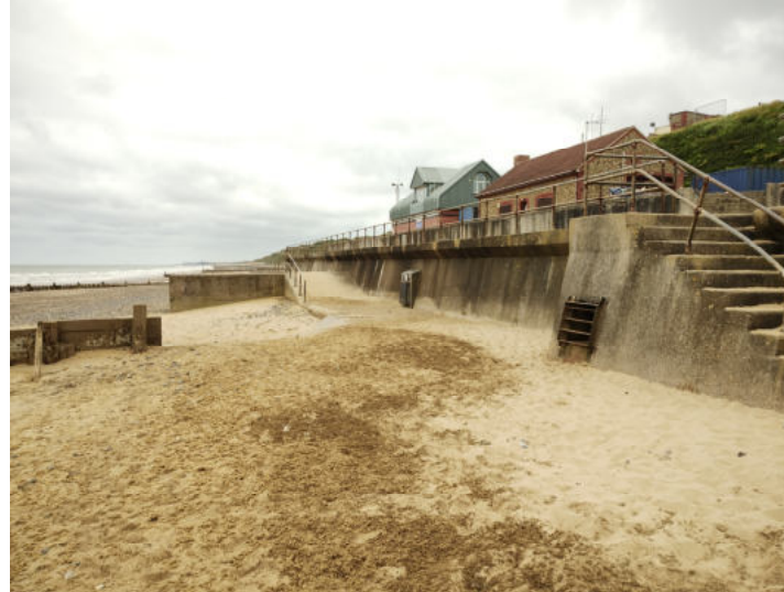
Recent view, showing elevated beach material and lower section of beach wall mostly submerged where the rocks would be placed against
