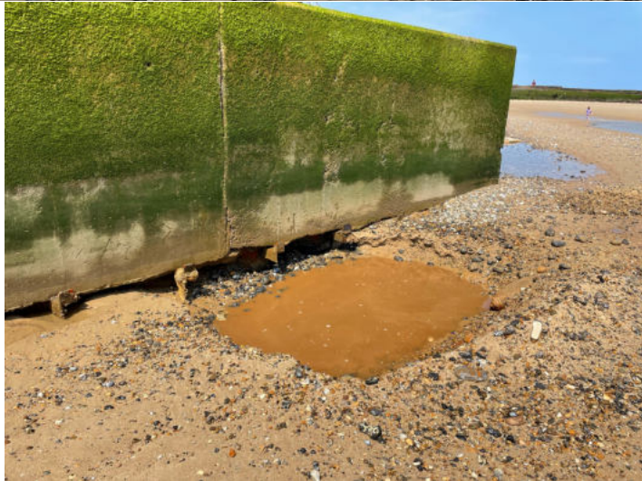
Older photos showing undermining of sea wall
