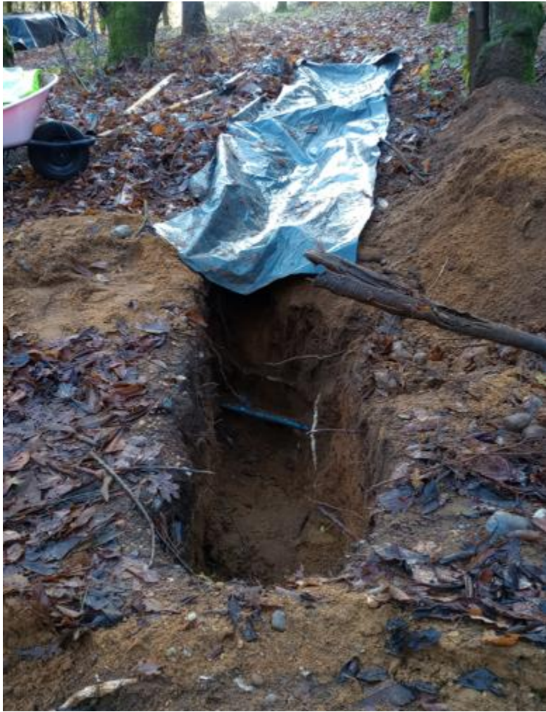
Water connection infrastructure
